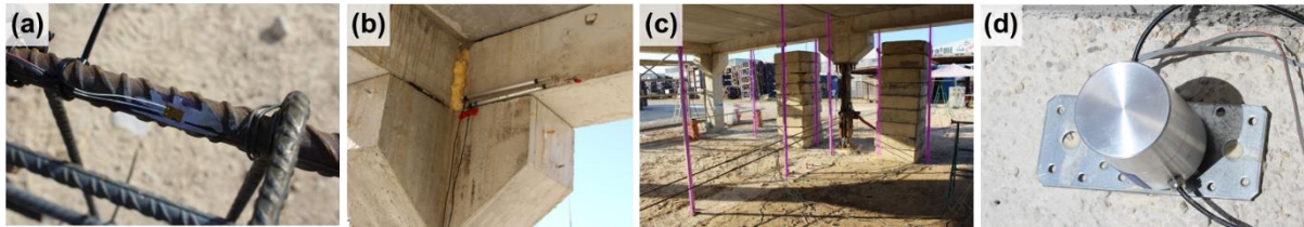
Figure 6. (a) Embedded strain gauge placed on rebar prior to being protected; (b) Horizontal displacement transducers; (c) Spring-loaded telescopic bars with transducers to monitor vertical displacement of first floor; (d) Accelerometer (All photos courtesy of Manuel Buitrago).
