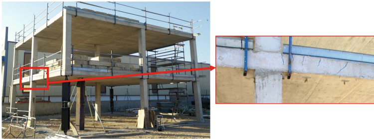
Fig. 5. Cracks on the slabs near the slab-column joint next to the failed column after its sudden failure.
