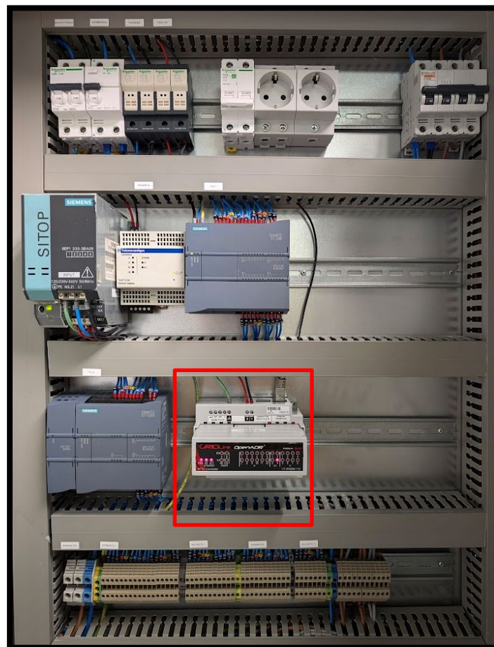
Figure 59: Installed hardware GRIDlink VT-IPM2M 113 series in the lab environment. Available at the e-SYM lab. Source: Own elaboration
