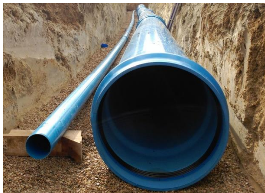
Figure 2.1. Pipes with different diameters.
