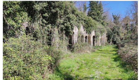
Fig. 3- The main front of the fort facing the high court yard invaded by the plants (Marinero, 2023).
