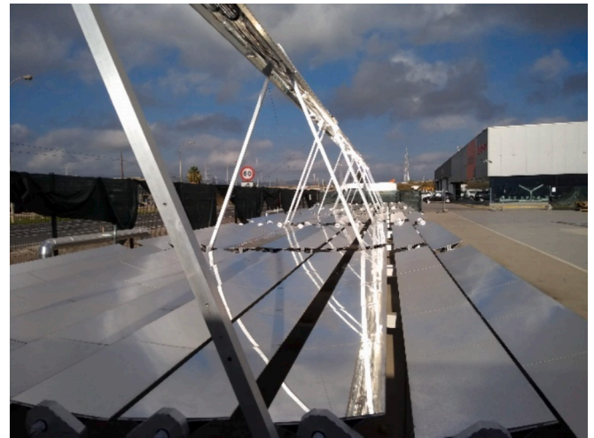
Fig. 2. Linear Fresnel collector modules solar field at the experimental site.
