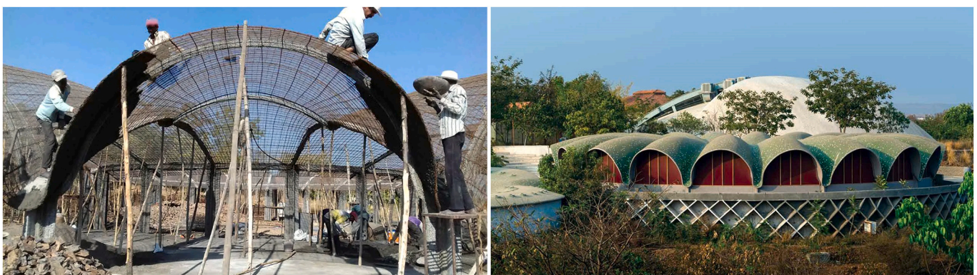
Fig. 3. Ferrocement building of Art of Living, Triveni Ashram, Pune, India; placing of mortar on steel mesh (left) and finished structure (right), ©Studio Acrobat.
