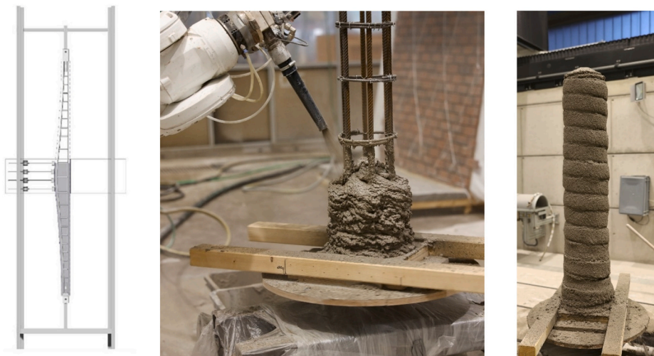
Fig. 19. Smart Dynamic Casting fabrication process with embedded reinforcement (left); and SC3DP of reinforced columns during (middle) and after (right) fabrication (©ITE, TU Braunschweig).
