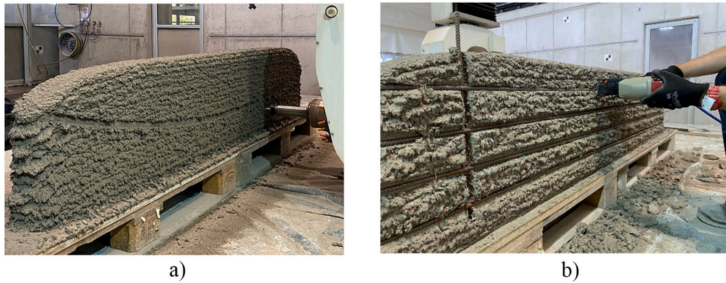
Fig. 21. Integration of force flow reinforcement through green state milling on SC3DP beam: a) robotic milling of force-flow optimised grooves, and b) integration of vertical and horizontal reinforcing bars; ©ITE, TU Braunschweig.
