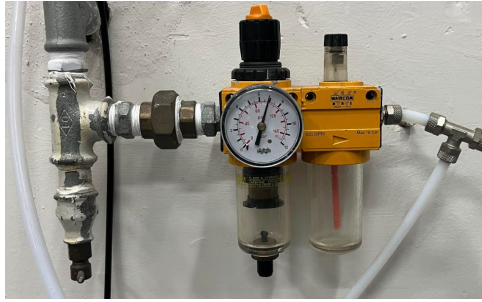
Figura 3.20. Manorreductor aire comprimido maqueta Cdm
