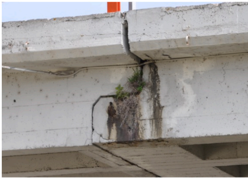
Fig. 1. Reinforced concrete dapped-end connection: overpass in road CV-500 near Valencia with deterioration due to diagonal crack at the re-entrant corner and poor state of the joint sealant.
