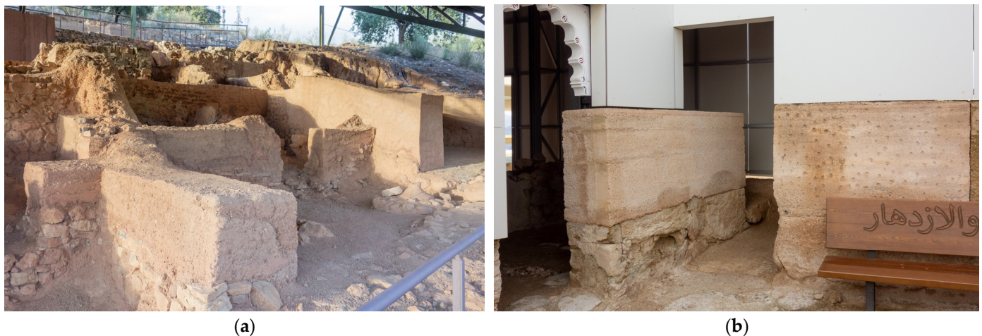
Figure 6. Intervention strategies and their carbon footprint: (a) volumetric reintegration of walls using adobe and nearby obtained materials in Cerro de la Cruz (Almedinilla, Córdoba); (b) reconstructions of elevations using colored concrete instead of earthen walls in Medina Siyasa (Cieza, Murcia).
