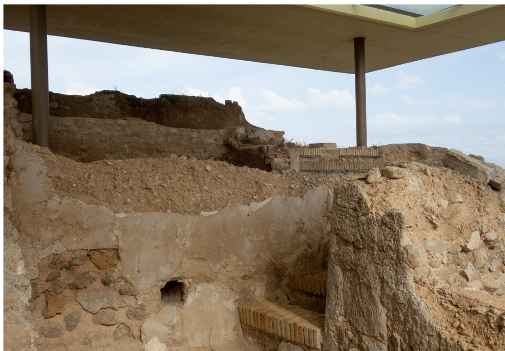
Figure 1. Partially collapsed rammed earth walls under contemporary protective cover at the archaeological site of Medina Siyasa (Cieza, Murcia).
