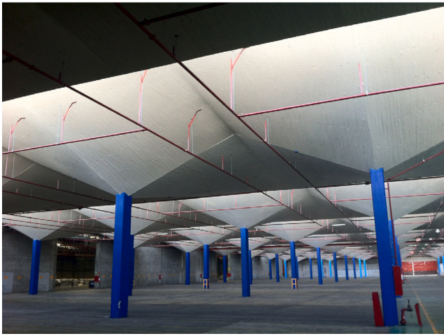
Fig. 2. Hypar umbrellas at the Bacardi factory near Mexico City. (Image: C. Lázaro).
