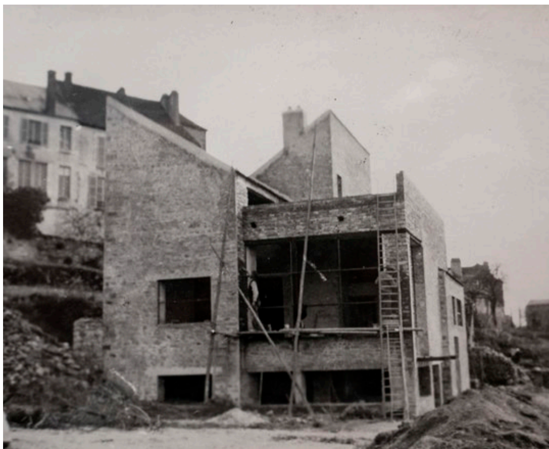
FIG. 40 Photograph of the Battanchon/Renaudin house from the North before the addition of the large cantilevered balcony, winter 1928-1929 (Bibliothèque Kandinsky).
