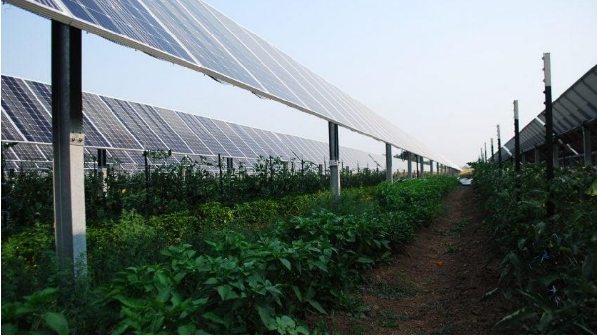
Figure 7 - Example of an installed agrivoltaics system (Dezeen.com)
