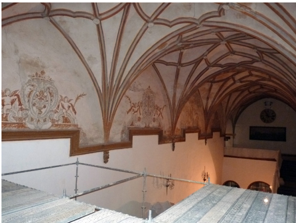
Fig. 11. View of the vault during the assembly of the interior scaffolding. (Source: Own elaboration).
