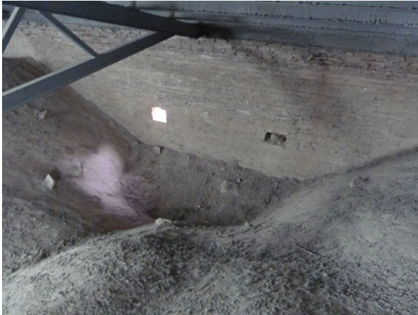
Fig. 10. Image of the extrados of the vaults during the restoration process. (Source: Own elaboration).
