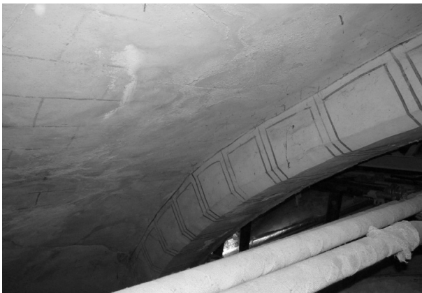
Fig. 14. Hidden arches in the false ceiling that were not removed during the 1970 intervention, when the wooden roof framework was replaced with metal trusses. (Source: Own elaboration).
