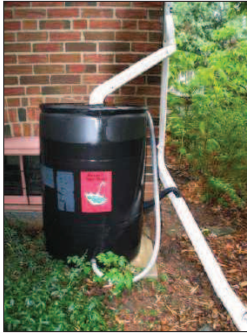
Figure 7.- Rain barrel. (TRC and CVC, 2010)
