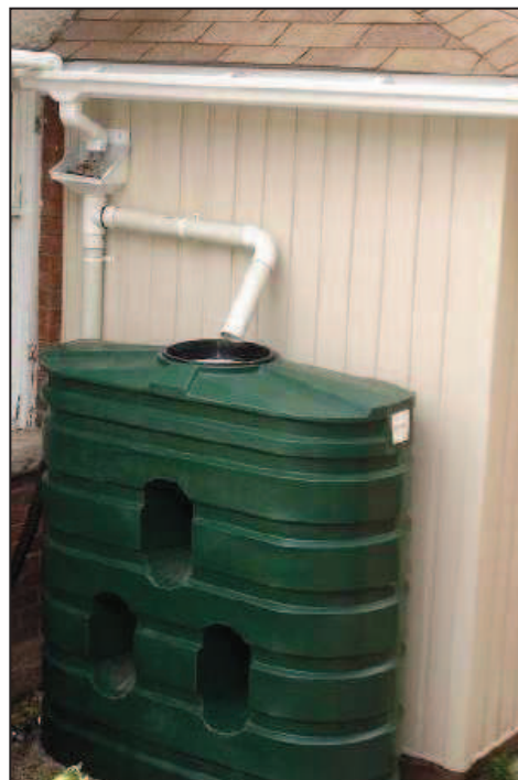
Figure 8.- Above-ground plastic cistern. (TRC and CVC, 2010)
