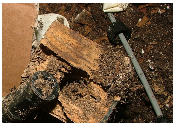
Figure 4. Node affected by termite activity.
