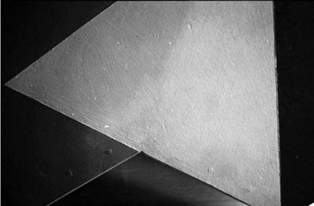
Figure 3. Detail of the cracks, deformations and lifting caused by the nail system used.
