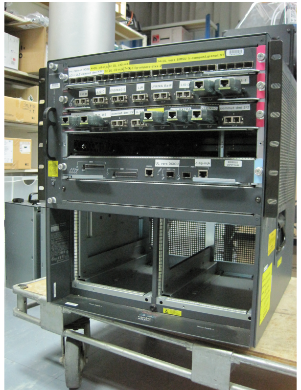
Illustration 16. Cat6506 already out of the rack, without the power supplies nor the FWSM since they are in the new chassis.
