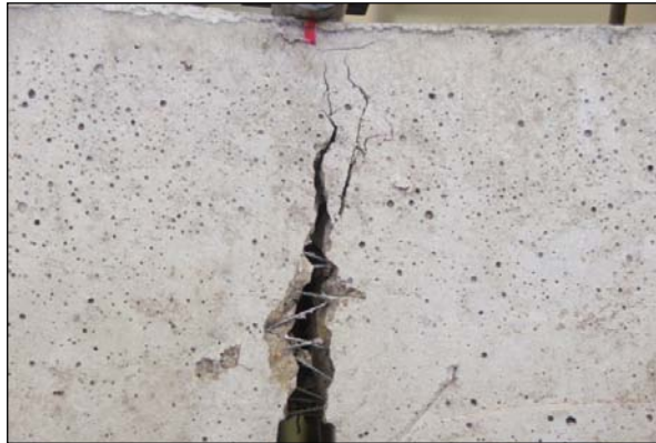
Figure 1.20. Sewing effect of fibers as observed in a cracked specimen right after being tested in bending.
