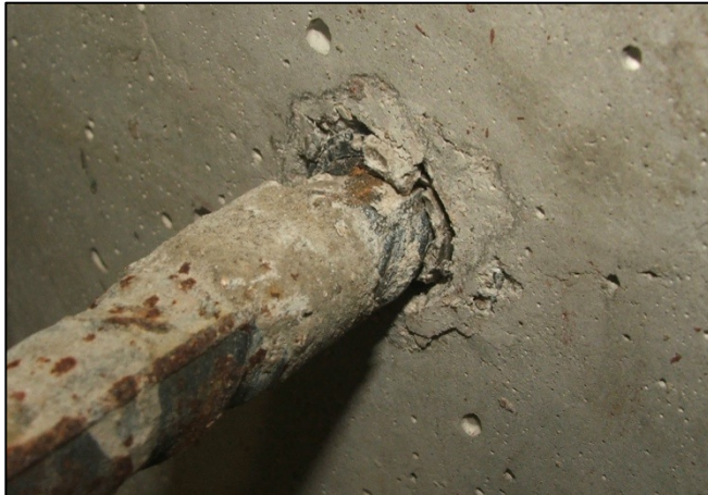
Figure 2.13. Example of pullout failure (detail).
