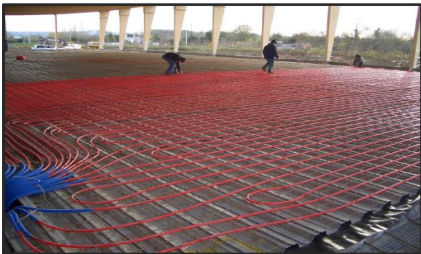
Fig. X. Picture of how will be the different circuits in Hall (22.1) area www.eurofast.ie
