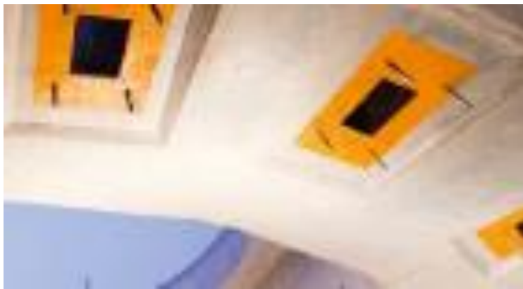
The tensors anchors
