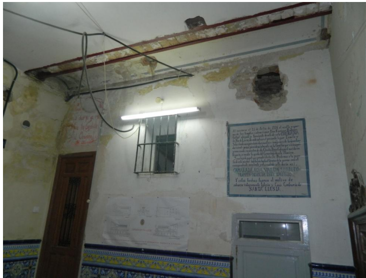
Picture 156. Inappropriate elements and mutilations
