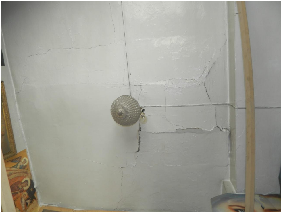
Picture 159. Craks in the gypsum ceiling
