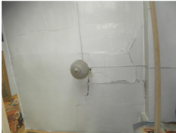
Picture 154. Fissures and cracks in the wattle ceiling
