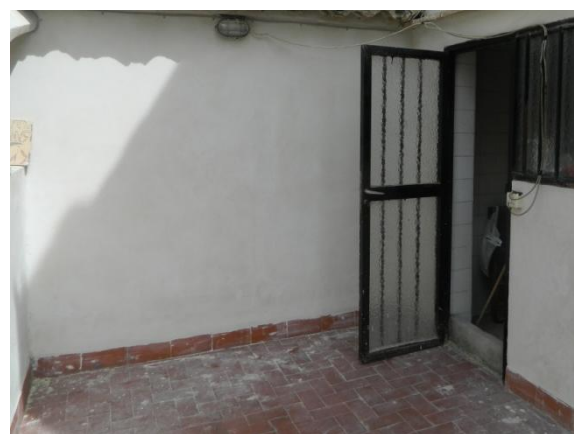
Picture 152. Passable plain roof where the filtration is produced
