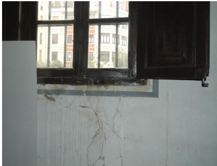
Picture 144. Vertical cracks under the window
