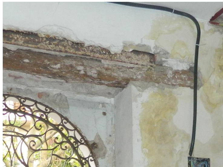
Picture 141. Metallic lintel bended over the Wood beam
