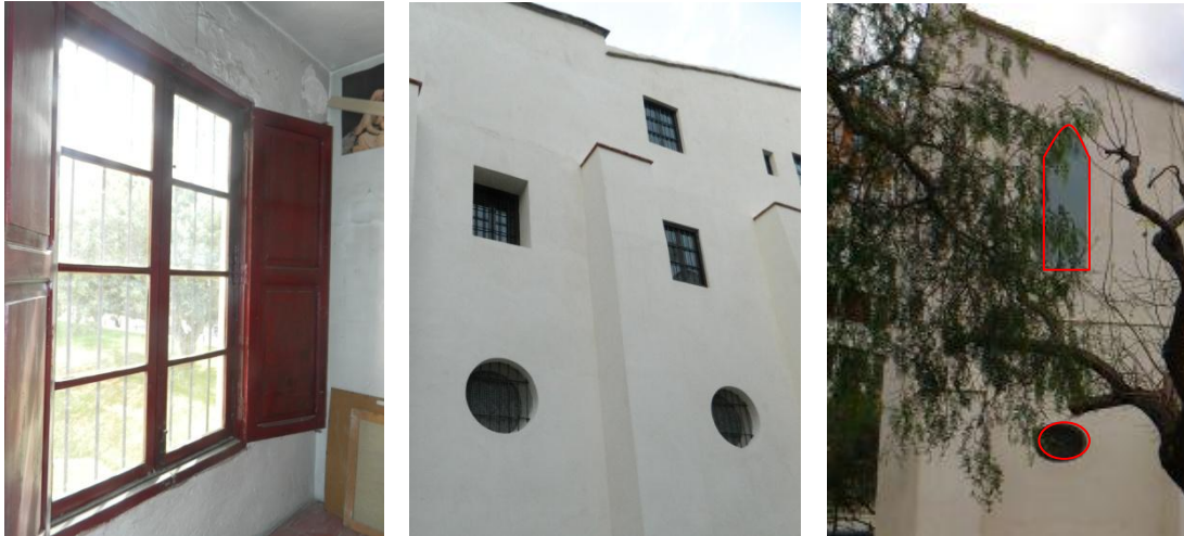
Pictures 124, 125 and 126. Different kinds of the Hermitage's windows. From left to right: rectangular, circular and oval shaped (5)
