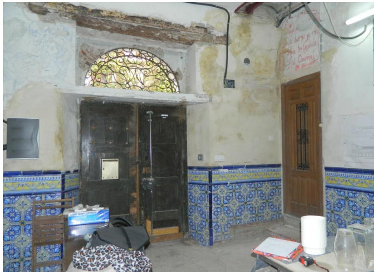
Picture 150. Filtration dampness
