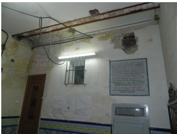
Picture 151. Filtration dampness
