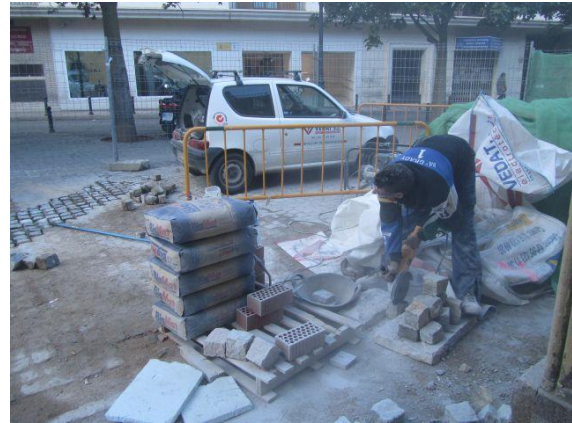
Picture 137. Sewage Works (47)
