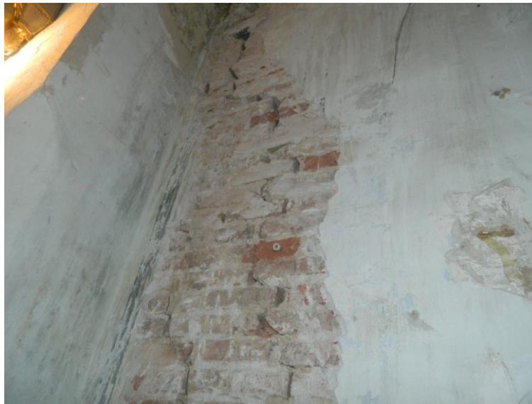
Picture 142. Vertical crack on the brick wall
