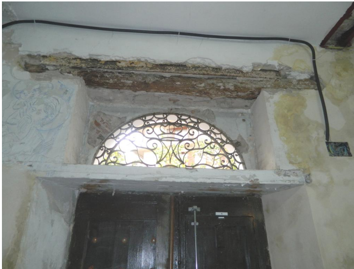
Picture 140. Loosening of the covering material
