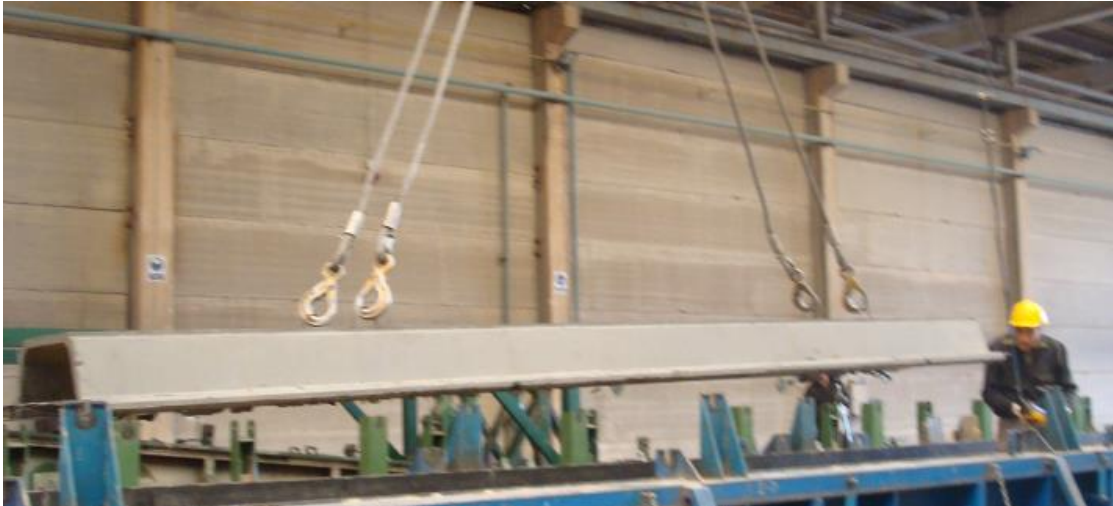
Figure A.4: Removal of a 5 meters length precast prestressed element 24 hours after casting
