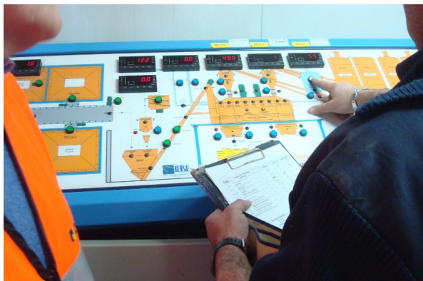
Figure 3.20: Control panel of the industrial mixer
