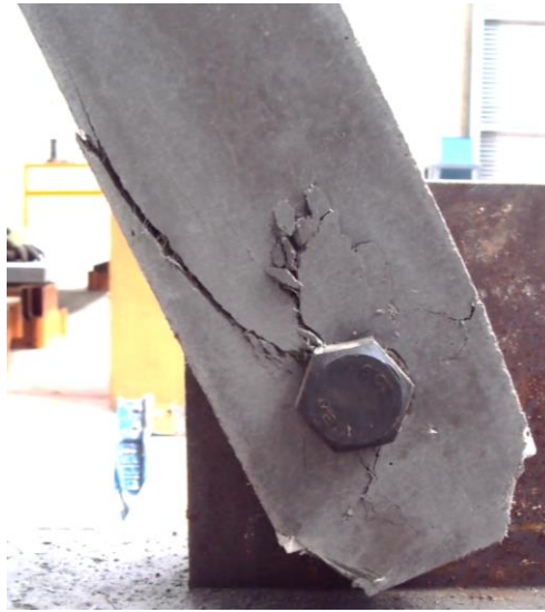
Figure 5.73: Joint of the compressive diagonal C5 after the bearing failure
