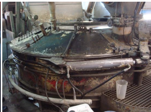
Figure 3.21: General view of the mixer
