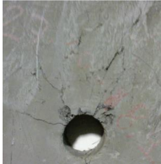
Figure 5.18: Bearing failure mode
