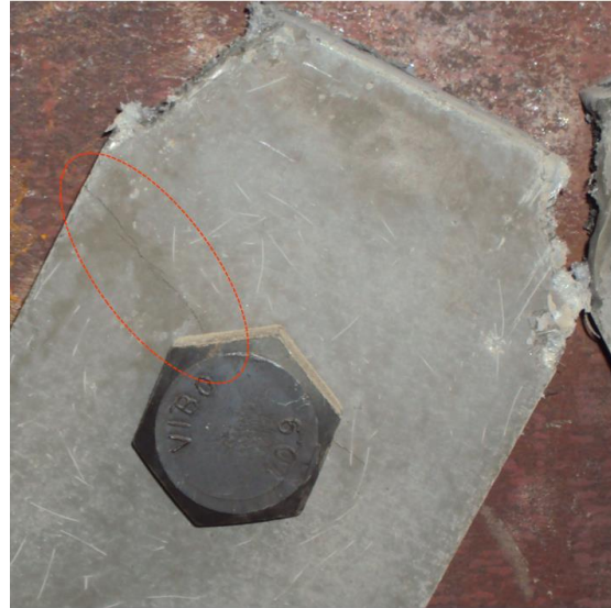
Figure 5.75: net tensión cracking at the upper joint of the diagonal T3
