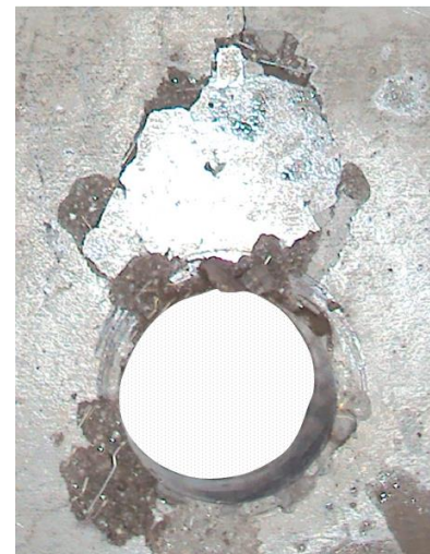
Figure 5.96: Example of bearing failure
