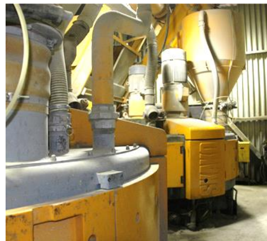
Figure 3.23: General view of the mixer
