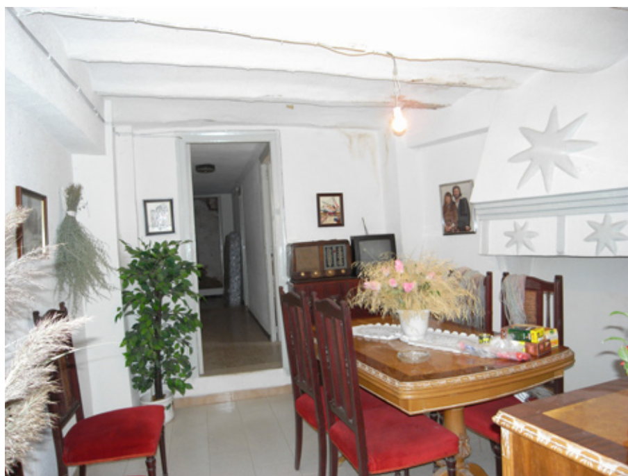
Photo4.1 The fireplace crosses the joists
