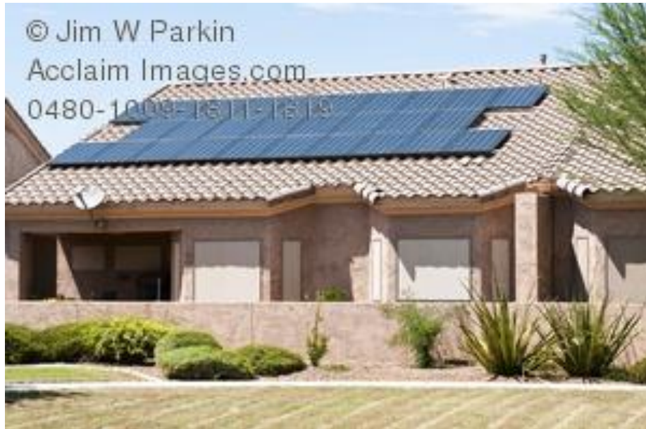
Figure 4. Roof mounted photovoltaic panels.
