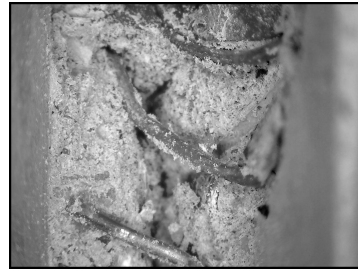
(b) Steel fibers sweeping the crack
