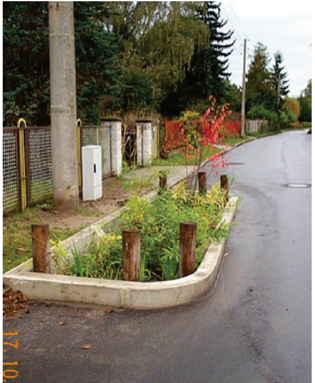
Figure 22. Rain garden INNODRAIN®
