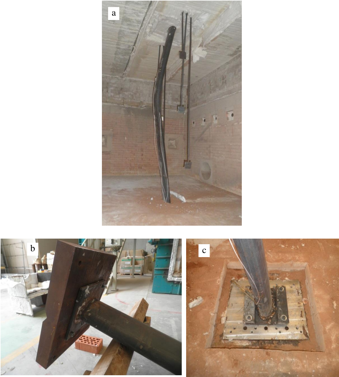
Fig. 5. Column after failure: a) general view; b) detail of the top end; c) detail of the bottom end
