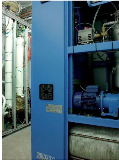
Ilustración 40.- BioSyngas/Wind to SNG. Container-integrated wind to SNG system with electrolysis stack and methanation device
