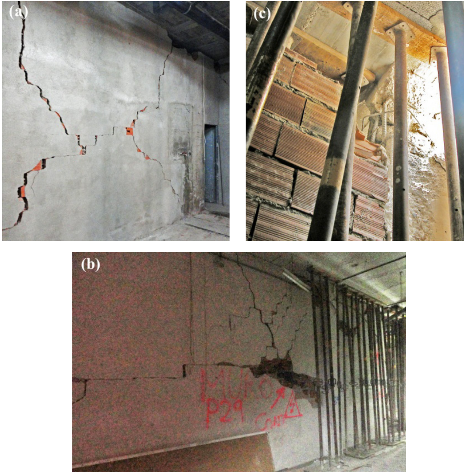
Figure 169: In-plane failures in masonry infill panels: shear diagonal cracking (a), horizontal sliding (b) and corner crushing (c)
