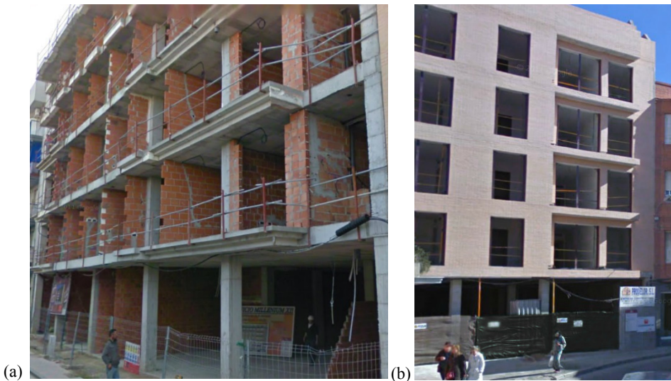
Figure 83: Examples of NCSE-02 typical buildings; likely high contribution of infills to the global strength and stiffness (a) and no compensation of infills reduction at 1 st storey by any increase of resistance of columns (b)
