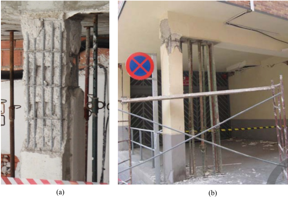
Figure 165: Damages in RC columns due to lack of shear-to-column (a) and column-to-beam (b) hierarchy of resistances
