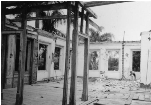
Figure 3. The destruction of Rialto Farm main house. Picture: José Roberto de Paula Barreira (1995).
