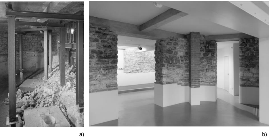
Figure 4. Restoration of the Music Pavilion of the eighteenth-century Villa Tatti Tallacchini at Comerio (northern Italy): a) during and b) after the intervention.
