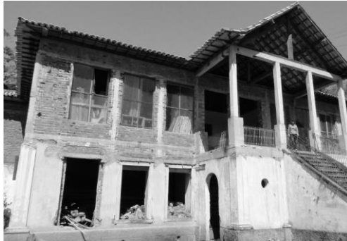
Figure 4. A spurious and unfinished rebuilding using bricks in the upper floor. Picture: Elizeu Franco (2013).
