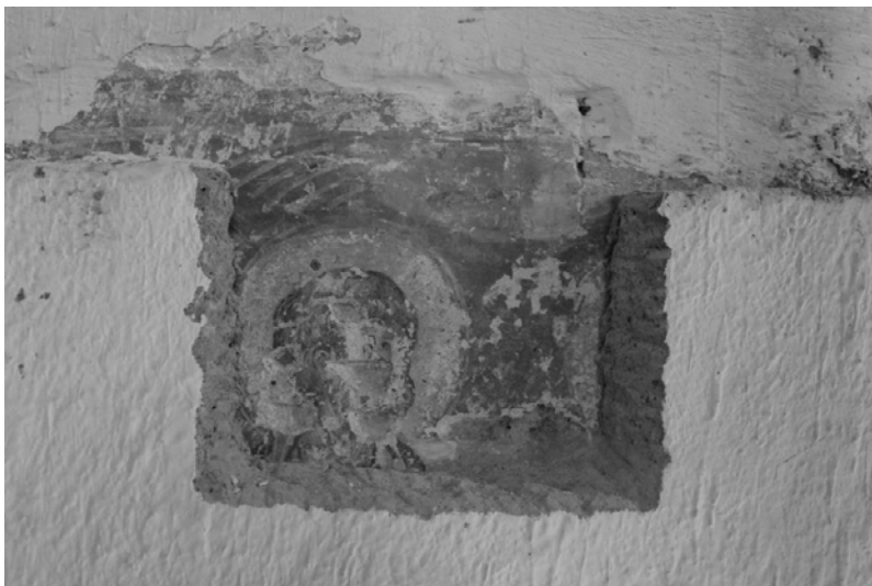
Figure 4. South wall (2nd bay) – lower register covered by cement-containing lime plaster. Trial 4 with a rather well preserved figure of the Pentecost panel.
