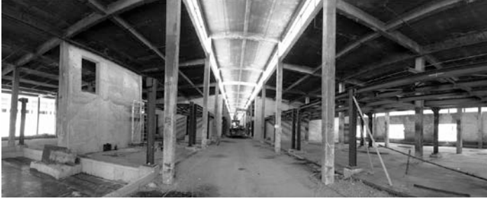
Figure 8. The restoration and re-use project for the Warehouse: interior space looking north through the central nave. (B. Asiliskender)
