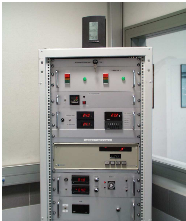
Figura 4.9 Caja de control (RACK).
