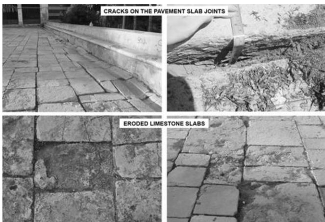
Fig. 8. Photographs of limestone slabs illustrating different degrees of eroding and cracks.
