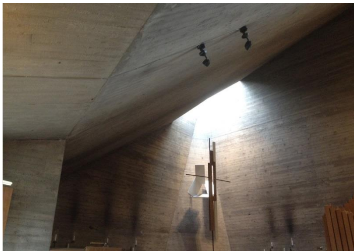
1. Interior of Västerort Church in Vällingby designed by Carl Nyrén and Bertil Engstrand, 1956.
