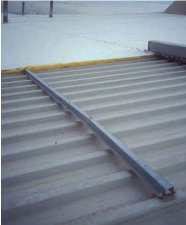
PANEL IN SITU
