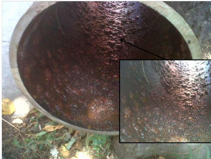
FIGURE 2.6: Metallic pipe with tubercles from the drinking water distribution system of Thessaloniki. Eva Ramos Martínez ©.
