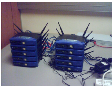
Figure 4: Typical router stack configuration.
