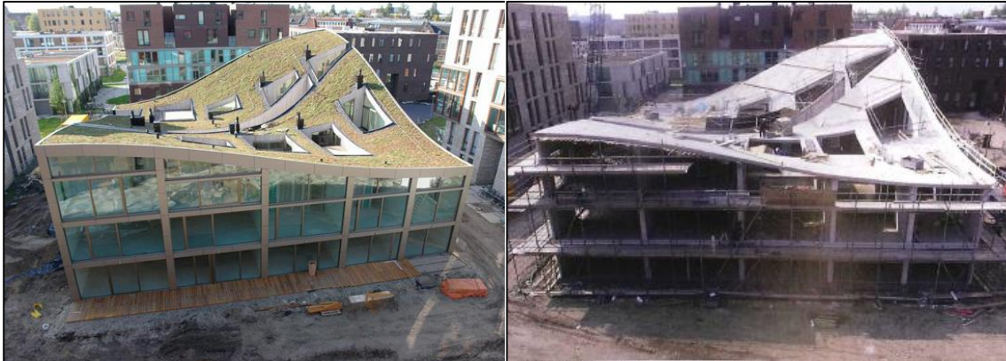
Fig. 26. Residential building “Het Funen” with curved cast in site roof (Amsterdam) (izda.) Detalle de construcción (dcha.)
