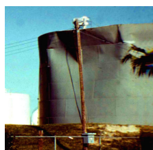
a) Windstorm buckling, USA
