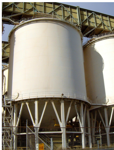
a) 10,000 tonne steel grain storages, Australia
