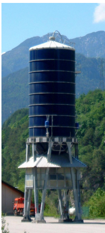
e) Salt storage with control room, Italy
