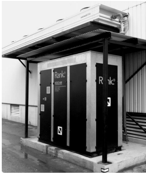
Fig. 2. ORC module and dissipation system [18].
