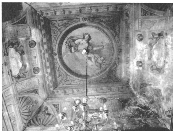
Figure 11: typical cracks in a segmental vault, Tomasoni, 2006)
