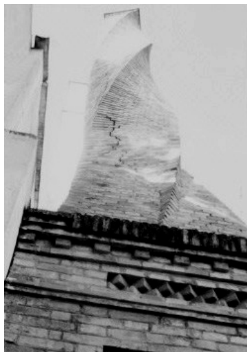
Figure 11. Distillery chimney by A. Bou Massana, Sant Quinti de Mediona, Barcelona, 1948 (Photo: Bou family archive)
