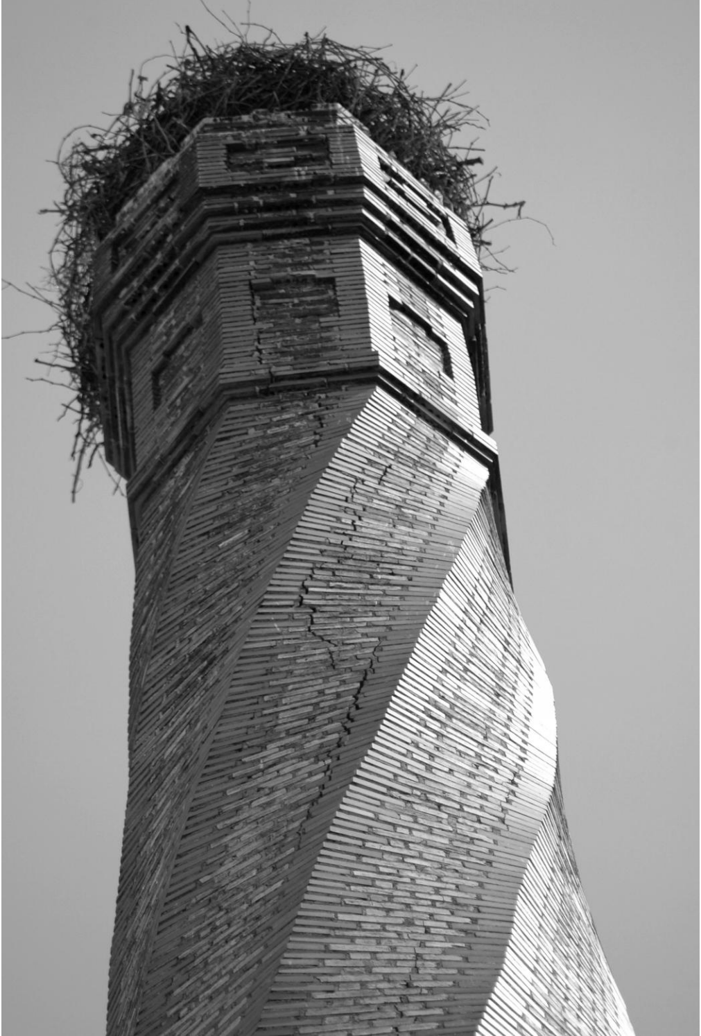
Figure 22. Detail of the intersection of the shaft and crown of the chimney, Tomelloso (Ciudad Real) (Photo: author)
