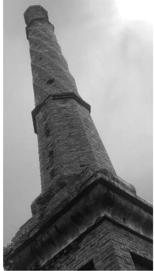
Figure 20. Chimney at Sanroma Mill (Baix de Monterol Mill), Reus (Tarragona) (Photo: Luis Rando & Lorena Escribano)
