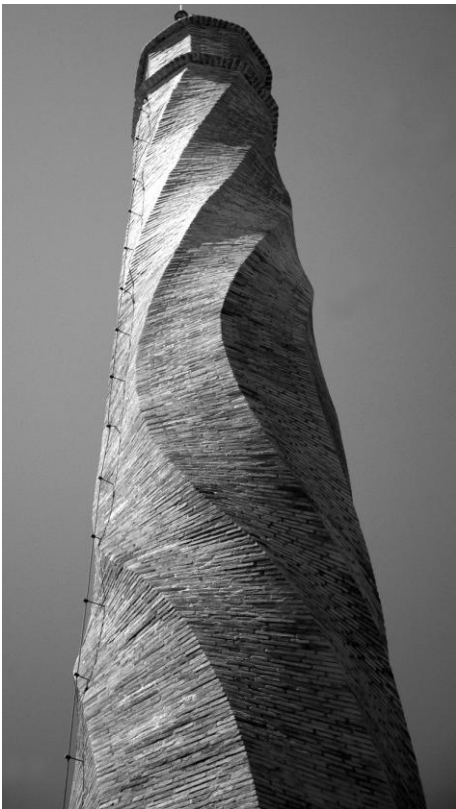
Figure 25. Double-twist shaft of Jose M. Granell ceramic kiln chimney, Alfara del Patriarca (Valencia) c.1910 (Photo: author)
