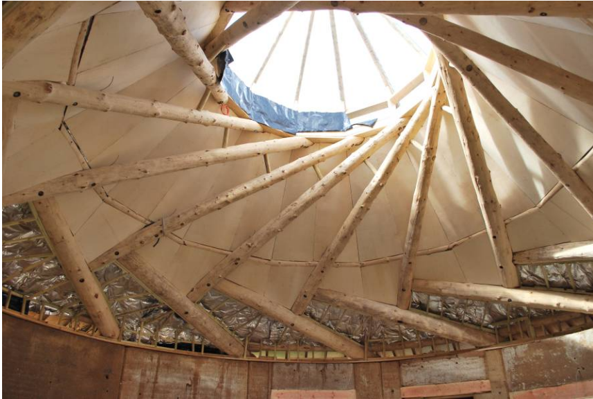
Figure 6: Internal view of the 'woven' reciprocal frame structure of the Woodland Community Hall. [Photograph: John Chilton]
