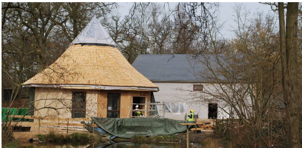
Figure 5: External view of the Woodland Community Hall roof nearing completion. [Photograph: John Chilton]
