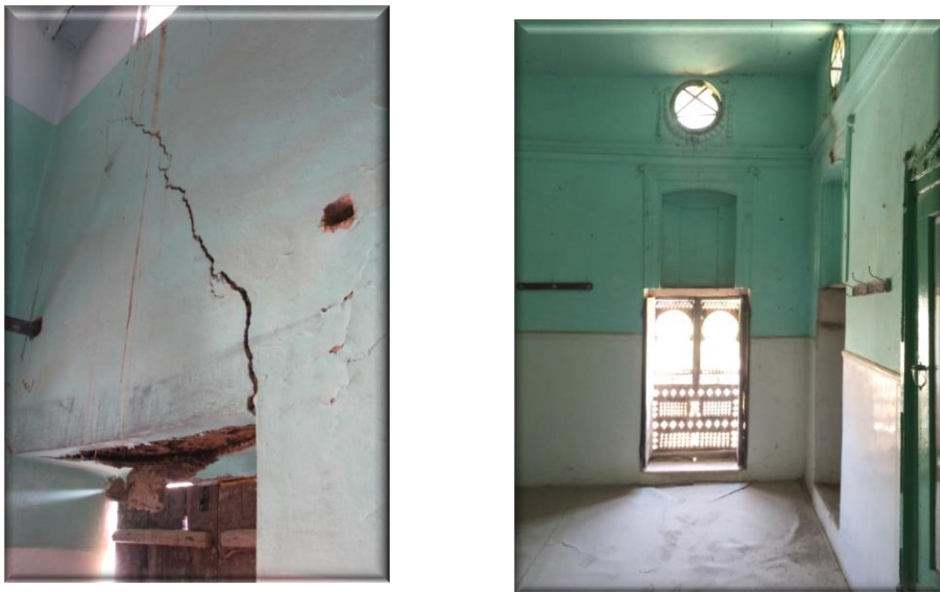
Figure 81. Cracked arched shelf within the Al-Junaid residence (Al-Aidarous,2014)
