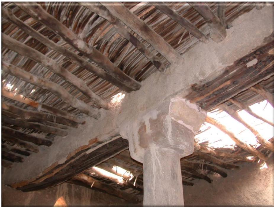
Figure 55. Decay caused by water and dampness (Al-Aidarous,2013)
