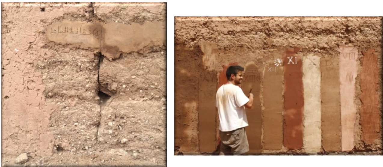
Figure 79. Cracks in the rammed earth at Talha, Testing different methods of rendering (Al-Aidarous,2014)
