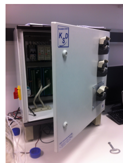
Figure 3. Control Box opened.
