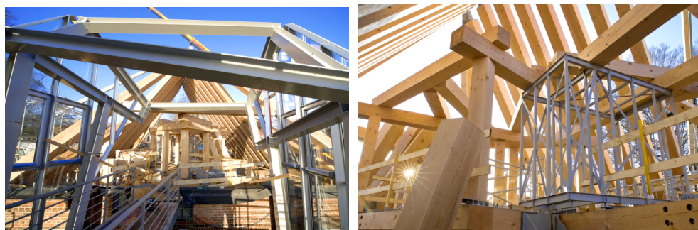
Figure 10: The Upper level under construction (a) stair house, and (b) meeting rooms
