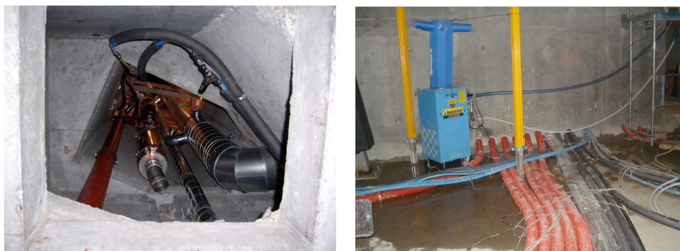
Figure 9: (a) Routing through fireplace and chimney, and (b) routing on foundation raft
