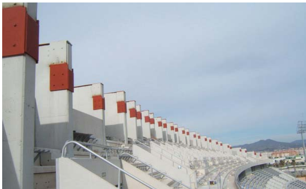
Figure 5. Anchorages prepared for the insertion of the grid. The new supplements are in red.
