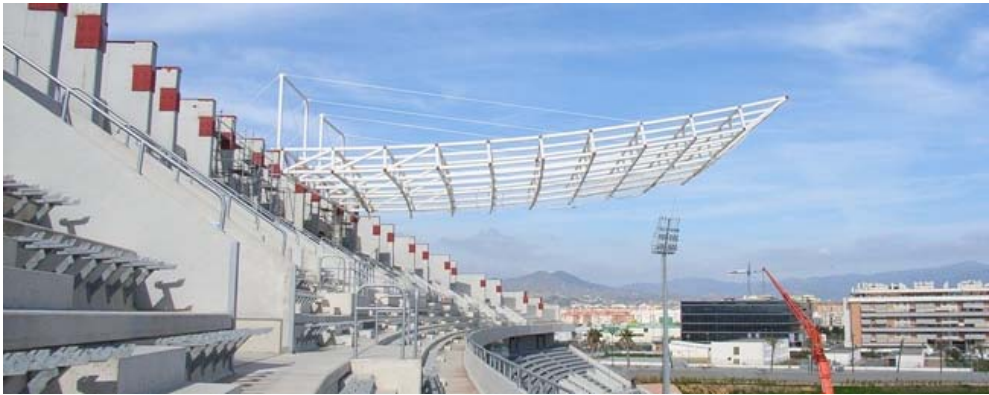
Figure 9. The cantilever was stayed provisionally with cables until we could complete the roof.
