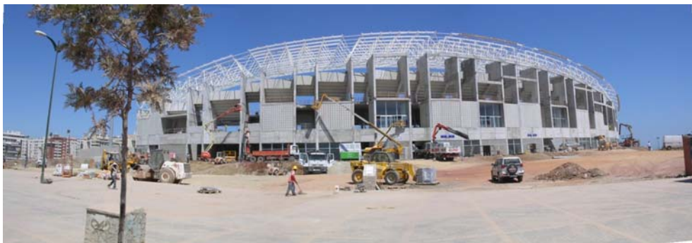
Figure 1. Spatial grid constructed with serious pathologies which led to its ruin.
