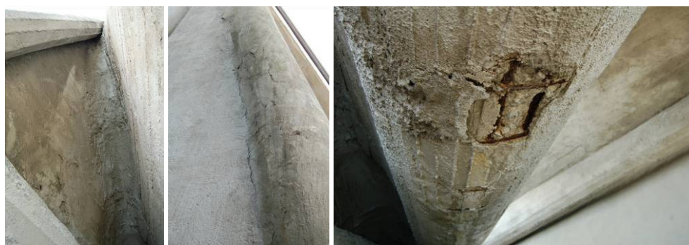
Fig. 15: present status of the building: a) internal point of extreme curvature of a vault, b, c) bar cover degradation.
