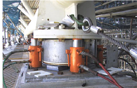
Photo 14: Jacks around a lead rubber bearing, Yamaguchi Dome (2000)
