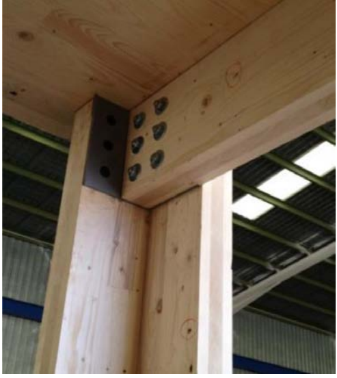
Fig. 4. Junction detail of the L-shaped support with the roof and the cross binding.
